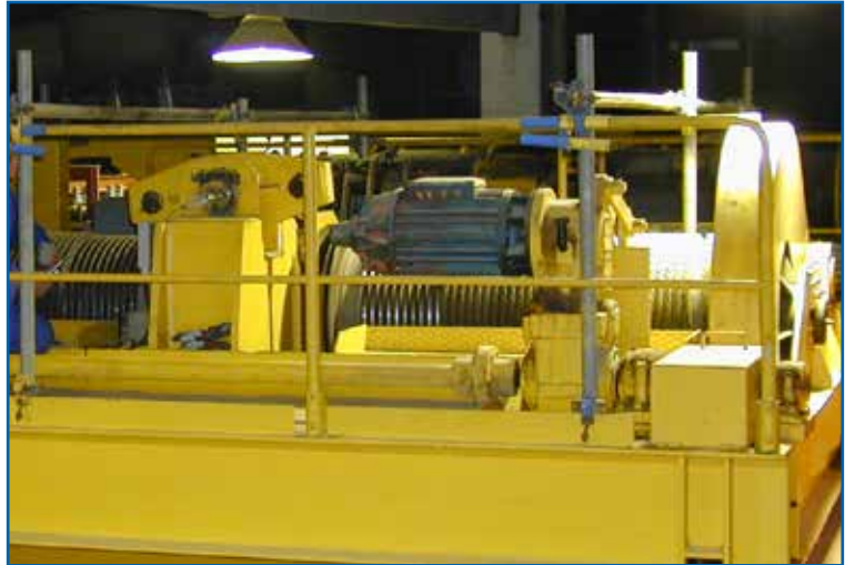
PIAB Load Pin SLC installed on a EOT as overload guard.
